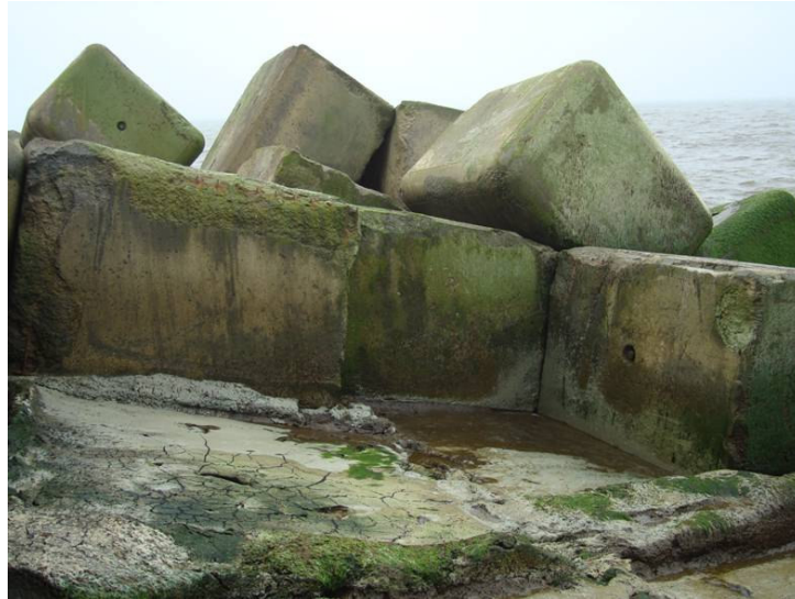
Figure 8. Cubes displaced from impermeable core at IJmuiden breakwater.
