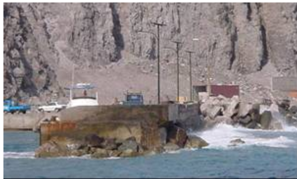
Figure 2: Saba breakwater after hurricane Lenny
