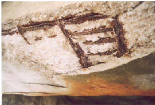
Fig. 1. Spalling at the base of a ramp over the tidal zone, the rest of the structure only shows mechanical damage.
