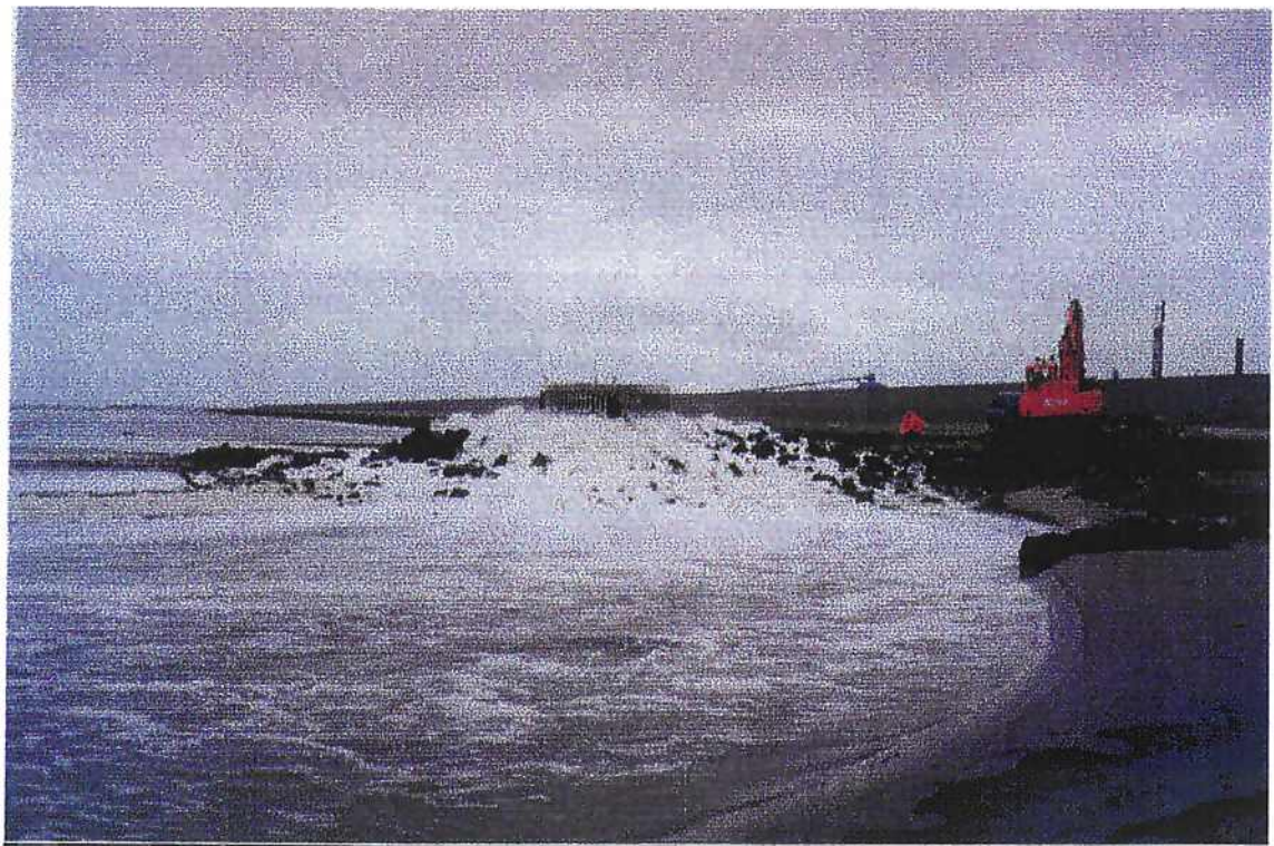
Figure 13 Outfall structure in operation
